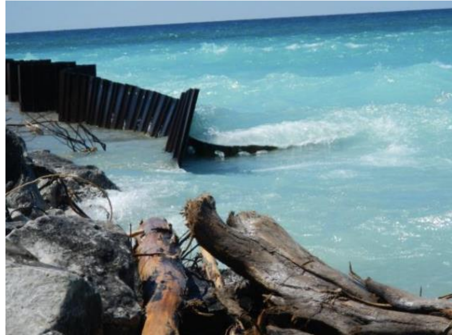
Extensive Damage to the Northern Steel Wall Visible
